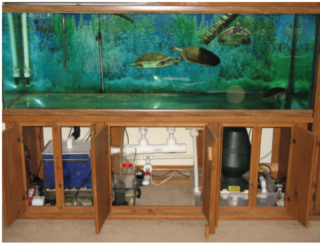
Water is treated with a UVC light, Bubble Bead filter, and trickle filter. The sump overflow is piped to sewer.
